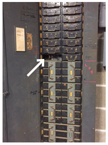
Herrick’s electrical panel is missing a breaker because a replacement no longer exists.
