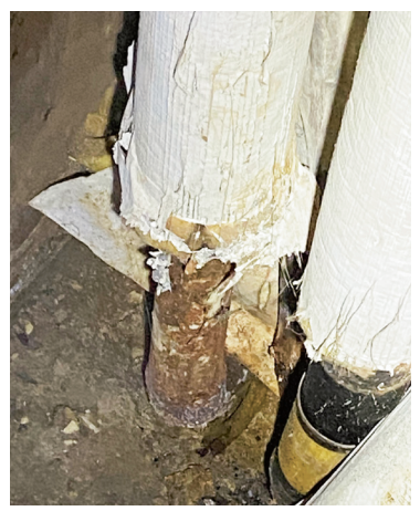
When this eroded water pipe burst in winter 2021, it caused heat failure and required emergency crews to work overnight on repairs.
