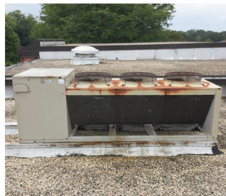
This summer, District 58 replaced Fairmount's 33-year-old condensing unit (pictured here) and 59-year-old unit ventilators with energy efficient models. The recommended life expectancy for a condensing unit is 15 years and unit ventilators is 30 years.
