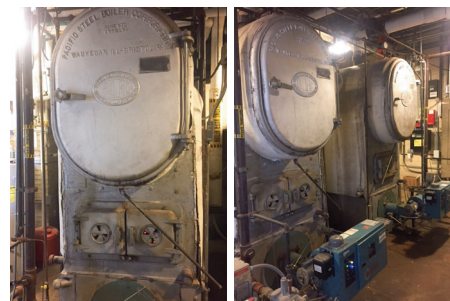
Pierce Downer's boilers, pictured here, are approximately 70 years old. The recommended life expectancy of a boiler is 30 years. The boilers are energy inefficient and very costly to maintain. This summer's HVAC work replaced these boilers.
